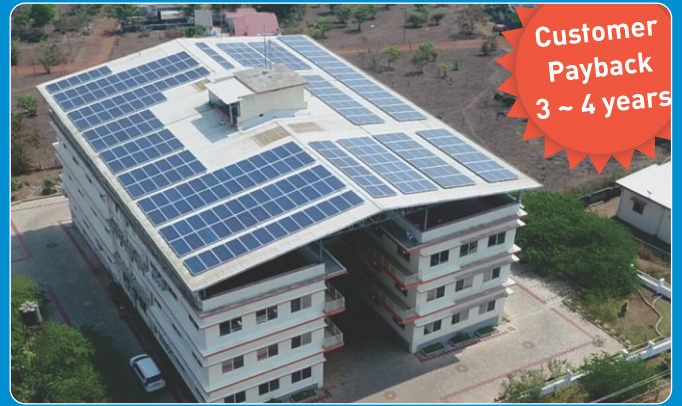
C&I Rooftop Solar Systems
